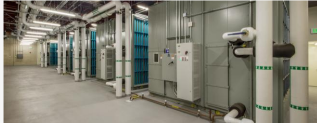
Cooling- and Thermal-Management Systems-
