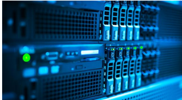
Servers and Routers
